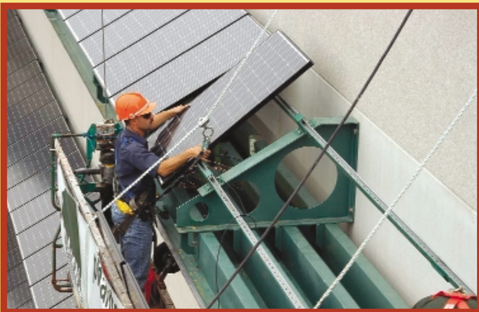
The HIT 190 solar panel from Sanyo. 189 panels were installed, covering a total of 222 square metres with a combined weight of 2,646 kg. A single panel, operating at 16.1% efficiency, can deliver a maximum output of 190 Watts of clean, green energy.
