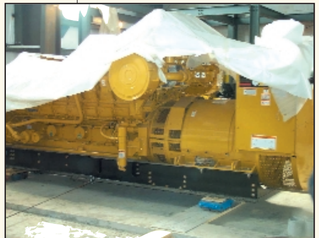
Each of the three engine generators will produce 925 kilowatts at Guelph's Renewable Energy Facility. (photo courtesy of Guelph Hydro Inc.)
