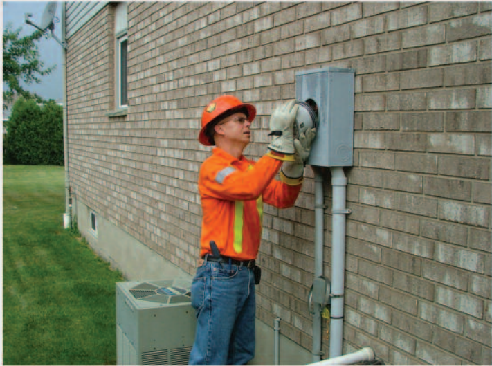
Meter installations tracked ahead of schedule and came in on budget. By December 2007 all residential customers had a new smart meter installed.
